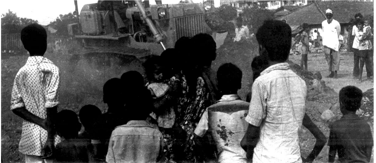
A black-and-white image of a bulldozer demolishing a slum in Mumbai, while some slum dwellers look on. Image from Anand Patwardhan's 'Bombay Hamara Shahar.' Courtesy of OVID.tv
